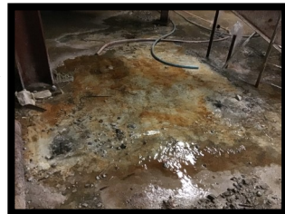
MS Basement Water Intrusion
