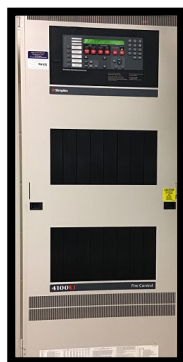
HS Fire Alarm System
