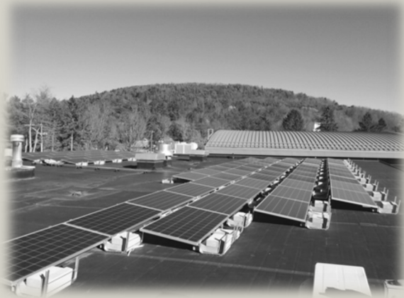
Middle School Solar Panels
